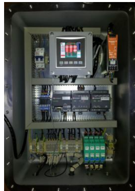
EX-D Electrical Panel
